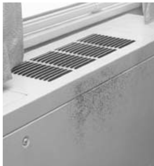
Mold growing on the surface of a unit ventilator. Moisture control is the key to mold control. If items are kept dry, mold does not grow.
